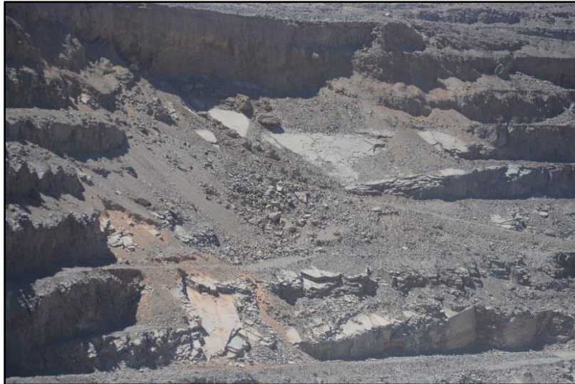
Figure 2: Planar failures on the Jwaneng mine eastern slopes mined with conventional vertical batters
